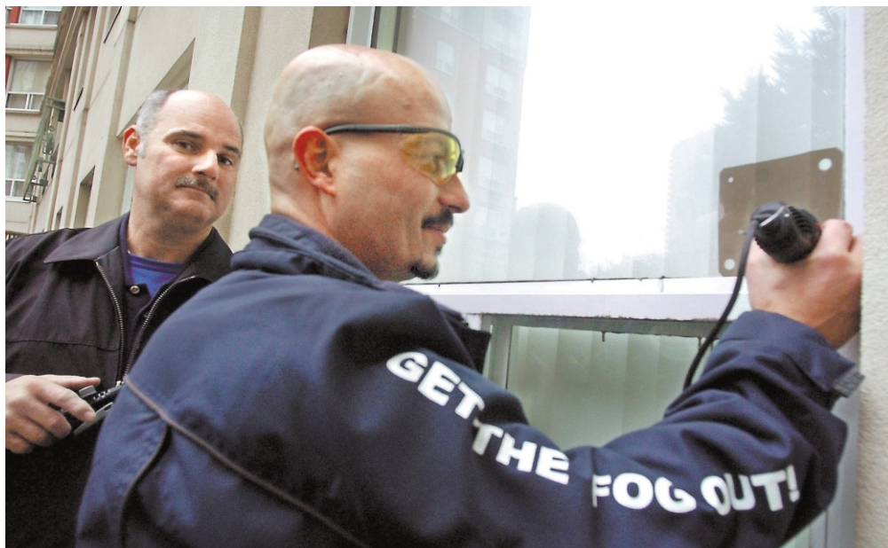
Sid Nayel, right, Eastern Ontario operations manager for Crystal Clear Window Works, makes repairs to a fogged thermal-pane window with Tom Conwayleft.
